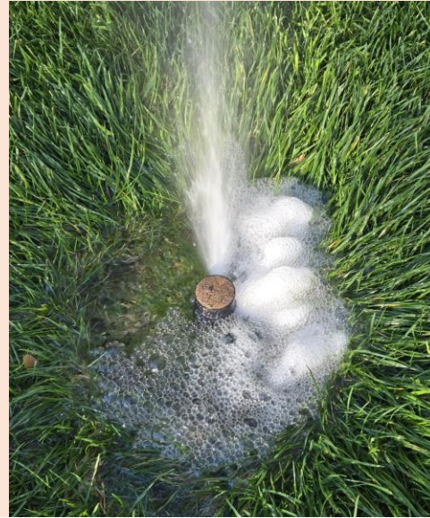
Sprinkler leak identified and repaired
