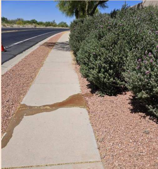
Leak detection during routine inspection
